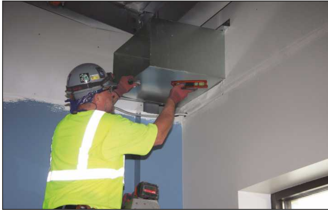
LEVELING A DUCT section at the Hannahville Indian Community’s new Governmental Services and Health Clinic Building is John Jacobson of Sheet Metal Workers Local 7. He’s employed by Berger and King.
