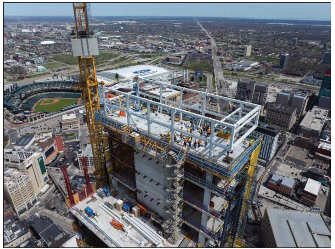
THE FINAL STRUCTURAL steel sections are seen atop the Hudson’s tower. Photo credit: Bedrock
